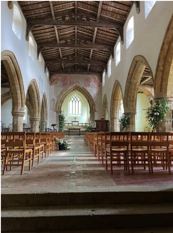
The sloping site is reflected in the three flights of steps from the west door to the sanctuary
